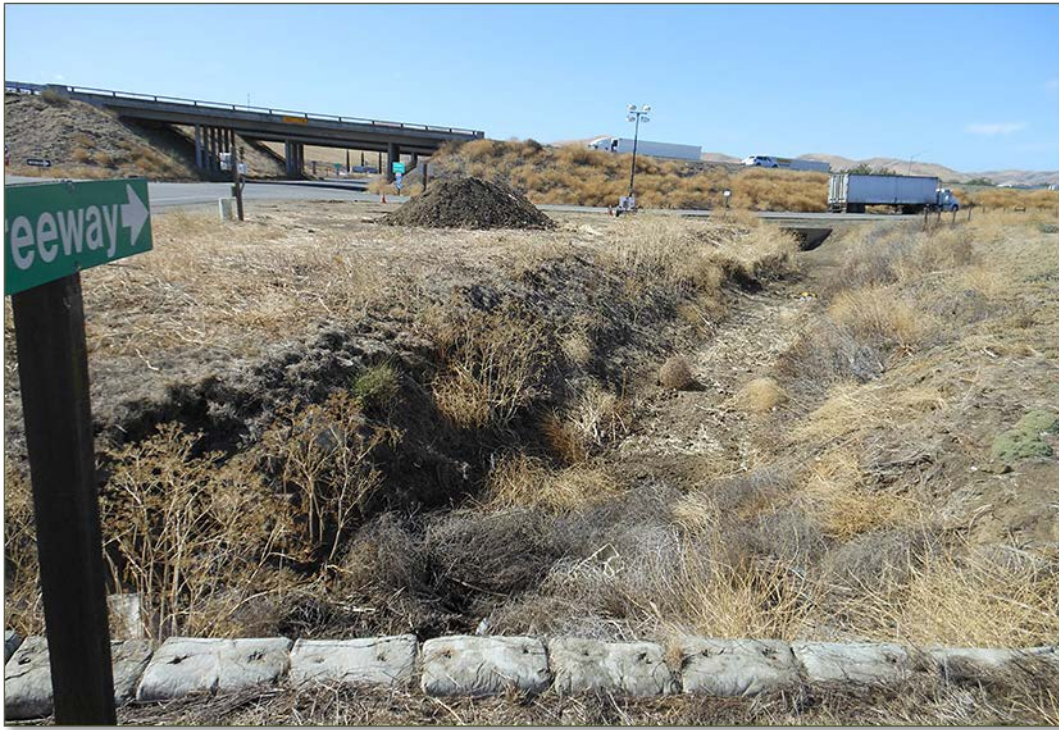
Realigned channel of Little Salado Creek (LSC4) along Fink Road east side of I-5.
