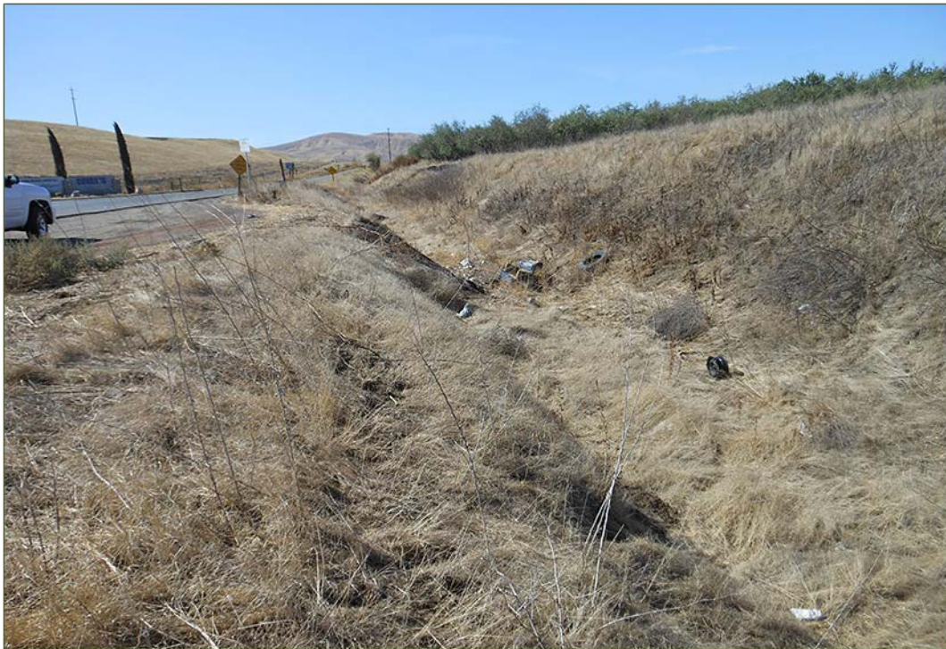
Realigned channel of Little Salado Creek (LSC5) along Fink Road west side of I-5.
