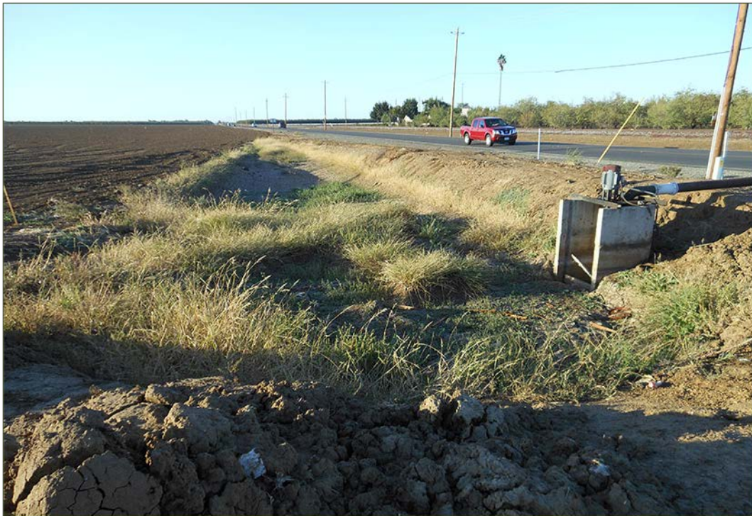
Agricultural ditch (D9) at intersection of Marshall Road and Highway 33 (sample point 3).
