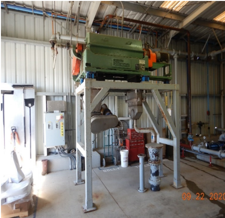
Photo No. 9: Decanter/dewatering unit.
