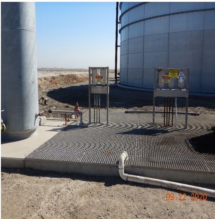
Photo No. 3: Influent lift station.
