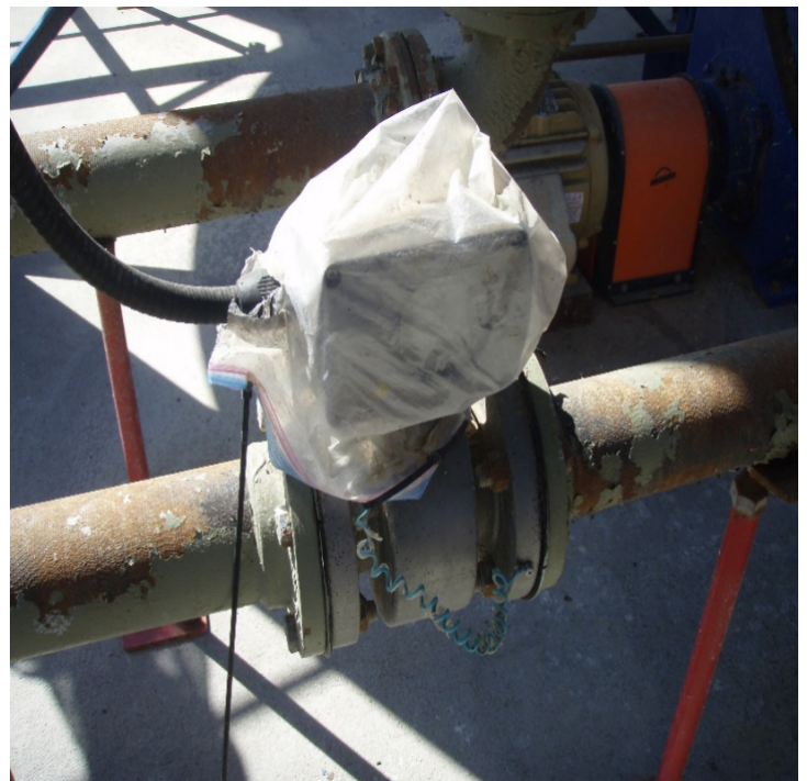
Photo No. 4: Influent flow meter.
