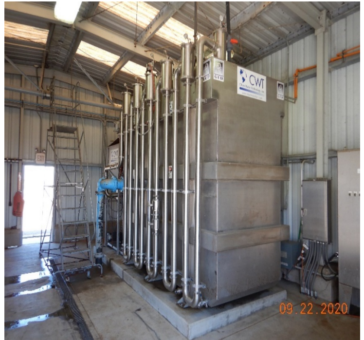
Photo No. 10: Clean Water Technologies, Inc – Gas Energy Mixing Flocculation and Flotation Unit.
