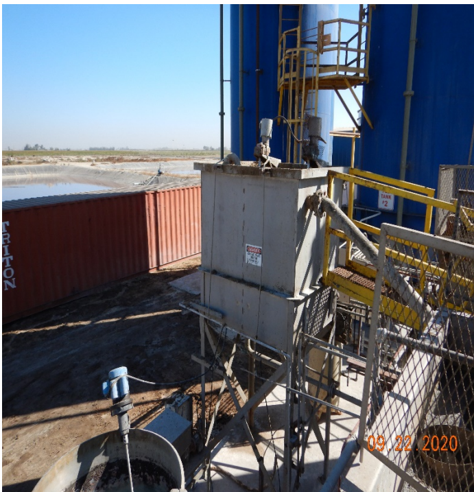
Photo No. 7: Flocculation tank at the treatment system.
