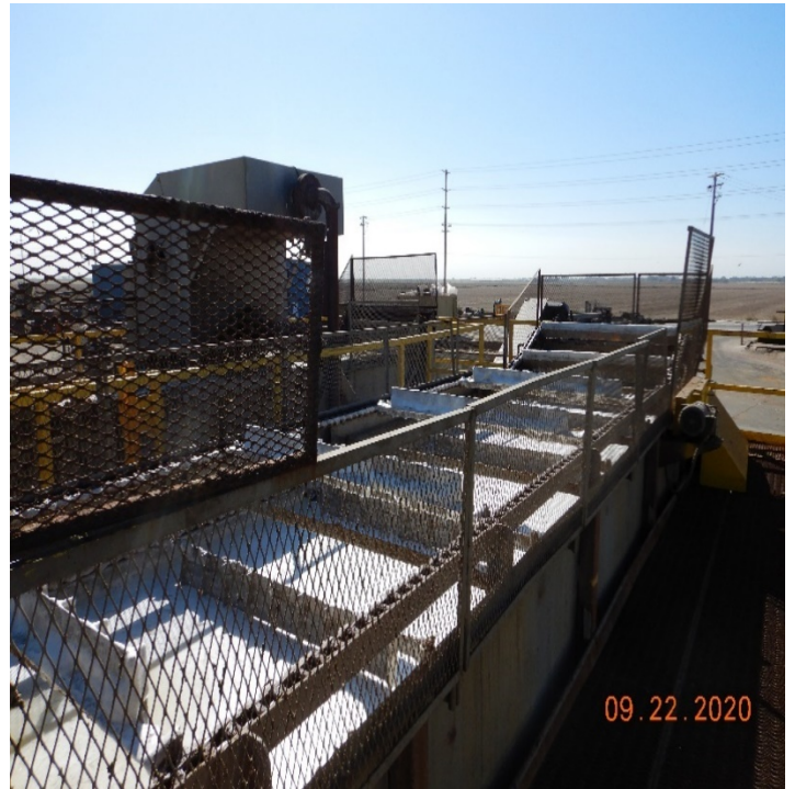
Photo No. 6: Dissolved Air Flotation Unit.
