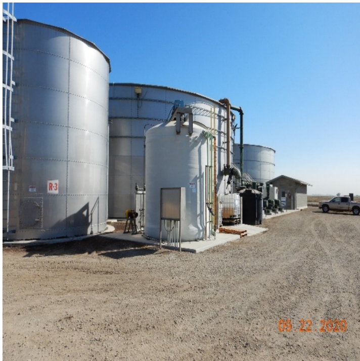
Photo No. 11: Bioreactor treatment tanks. The small tank contains magnesium hydroxide.
