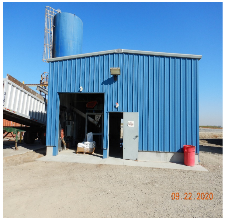
Photo No. 8: Building containing the decanter/dewatering unit and Gas Energy Mixing Flocculation and Flotation Unit.
