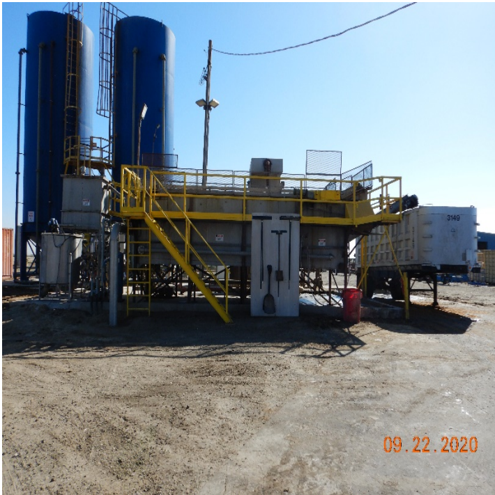
Photo No. 5: Wastewater treatment system.
