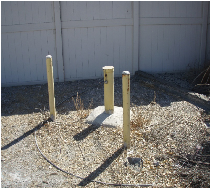
Photo No. 23: One of the groundwater monitoring wells at the facility.
