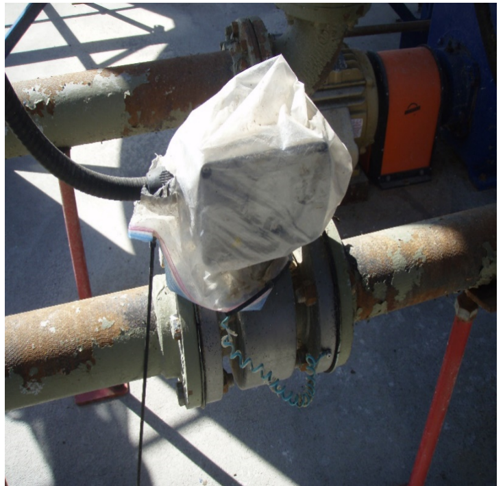
Photo No. 4: Influent flow meter.
