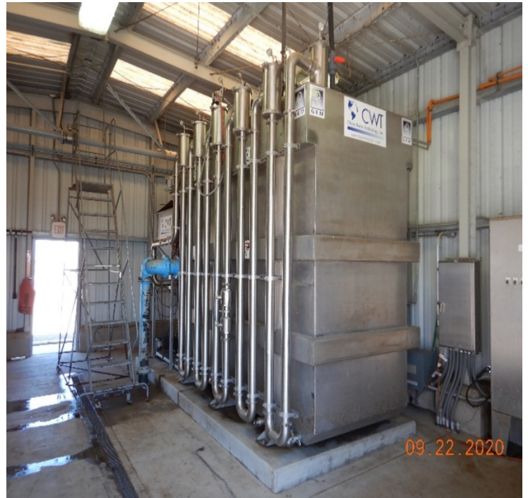
Photo No. 10: Clean Water Technologies, Inc – Gas Energy Mixing Flocculation and Floatation Unit.
