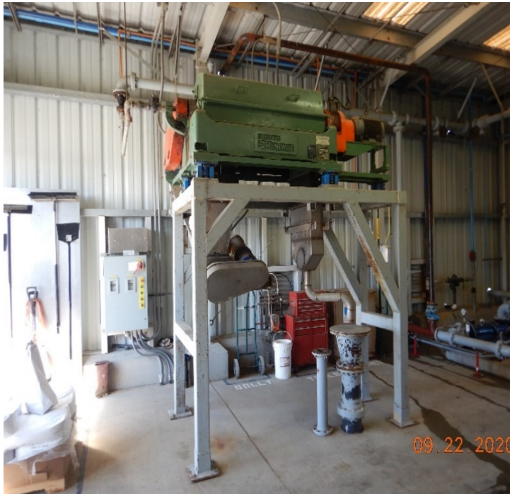
Photo No. 9: Decanter/dewatering unit.
