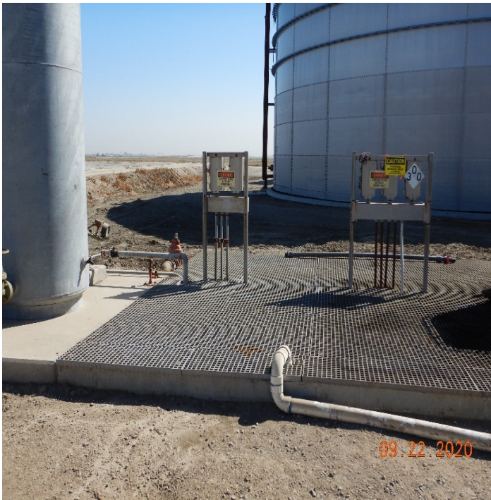
Photo No. 3: Influent lift station.
