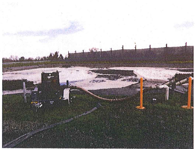
Figure 8 Looking at an additional pump along the East Pond. This pump is used to supplement existing pumps to transfer leachate to the West Pond.
