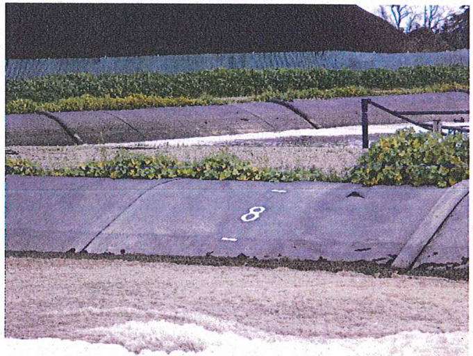
Figure 10 Looking at the freeboard marker in the Treatment Pond. Over 2 feet of freeboard was available.
