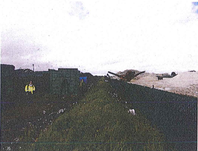
Figure 11 Standing east of the Raw Compost Receiving and Processing Area, looking northwest/upstream along the eastern leachate control berm.
