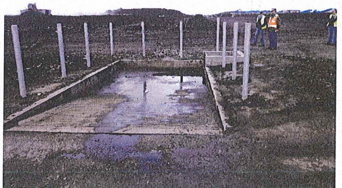
Figure 30 Looking northwest into a Catch Basin D along the central drain, that is located between the finished Phase 2 and 3 composting pads.
