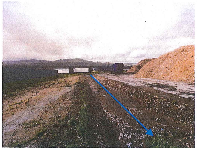
Figure 20 Looking west along the western leachate drainage channel, the blue arrow show the leachate flow path.
