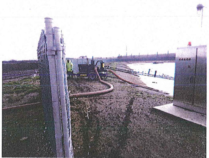
Figure 16 Looking at an auxiliary pump that was being used to transfer leachate from the West Pond to the tanker truck in Figure 17.
