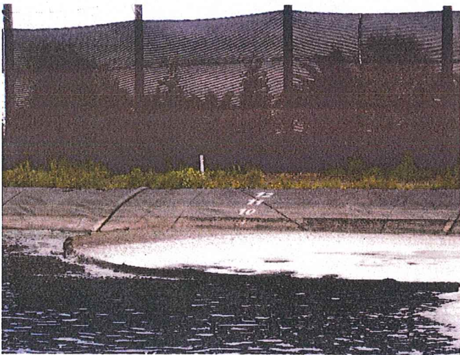
Figure 7 Looking east at the East Pond's freeboard marker. Over 4 feet of freeboard was available.
