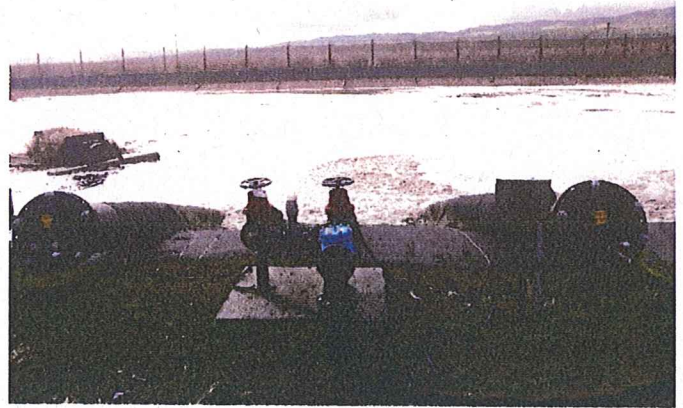
Figure 14 Looking south across the West Pond. Only two of the ponds three aerators were operating.
