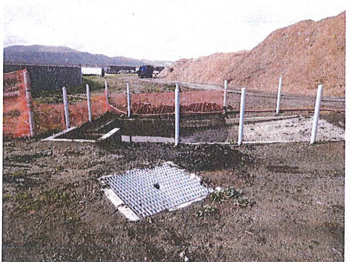
Figure 18 Looking west at the southern most catch basin along the central drain. This is the last leachate catch basin/drain prior it discharging into the West Pond.
