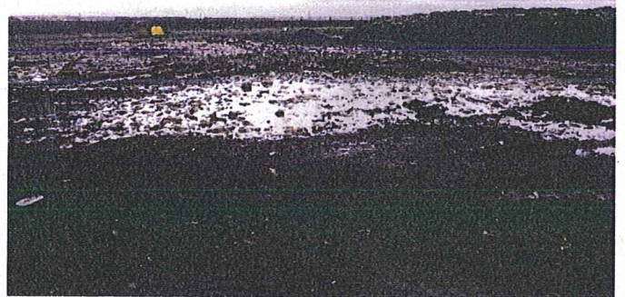
Figure 34 Ponding just south of the Raw Compost Receiving and Processing Area, atop a yet to be finished composting pad.
