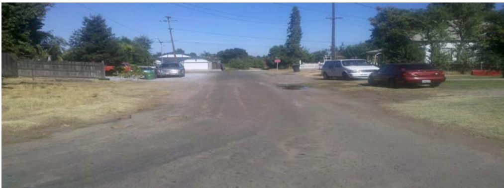
Photo reflects La Gallina Chicken Avenue in need of curb, gutter, storm drain, sidewalk, and street repaving.
