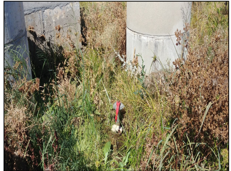
Leaky Pipe Near Sample Point 5, September 24, 2019
