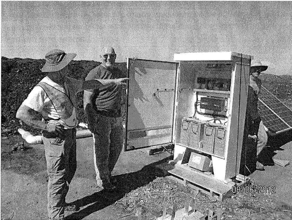
Photo 8: Interior of the power array box. From bottom to top: batteries, inverter, timer and switches, and exhaust fan at very top. From left to right: Harold Ruppert and Peter Moon of OZ Compost, and Kevin Barnes, City of Bakersfield.
