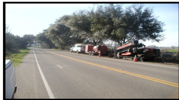
Typical Orange Blossom Road encroachment
