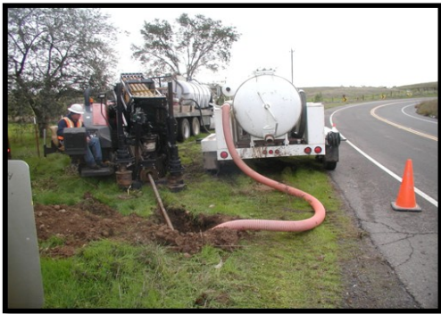
New Fiber Optic cable brought to his- toric Knights Ferry from Oakdale through Rodden Road
