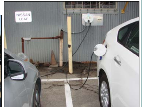
Electrical Docking Station
