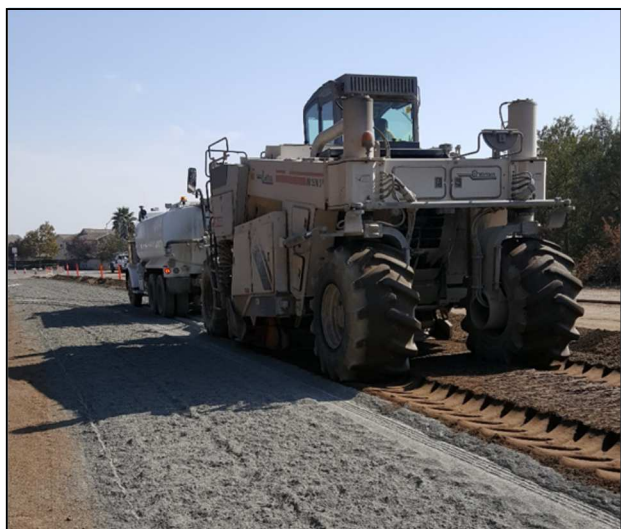
Top Photo: Howard Road Paving Bottom Photo: Soil Mixing on Hatch Road
