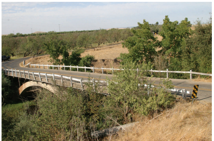
Tim Bell Road Bridge over Dry Creek — Reinforced concrete arch bridge with a wooden superstructure, which is maintenance intensive.
